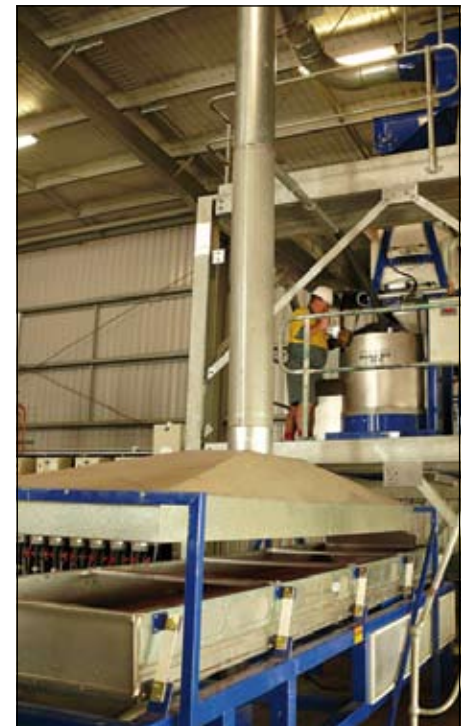
The centrifugal batch mixer — part of the new seed treatment plant.
