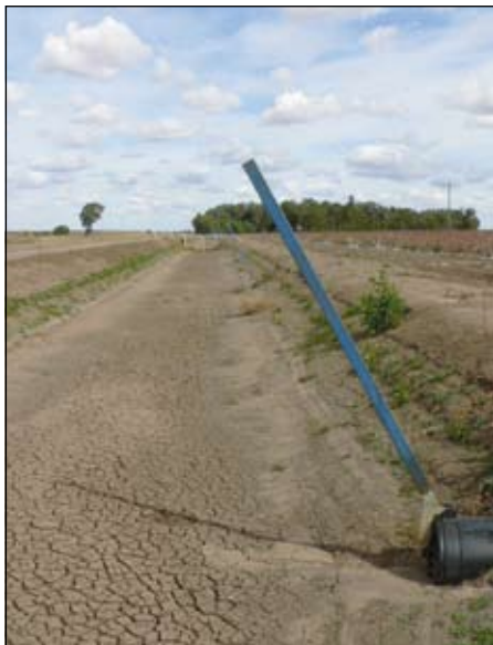
The pipe through bank system.
