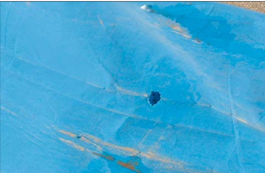
Typical vermin damage — showing the need for doming modules.
