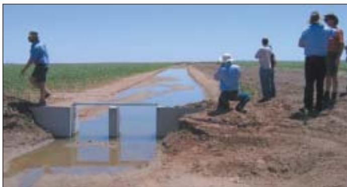
Looking downstream on the large 200 x 500 metre bays. Culvert capacity is 60 megalitres per day of supply water plus drainage water from the upstream bay. Note the ease of access from the raised roadway to the culvert.
