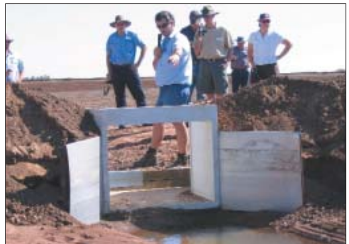
Large capacity culverts are required to handle the high flow rates of combined supply and drainage.
