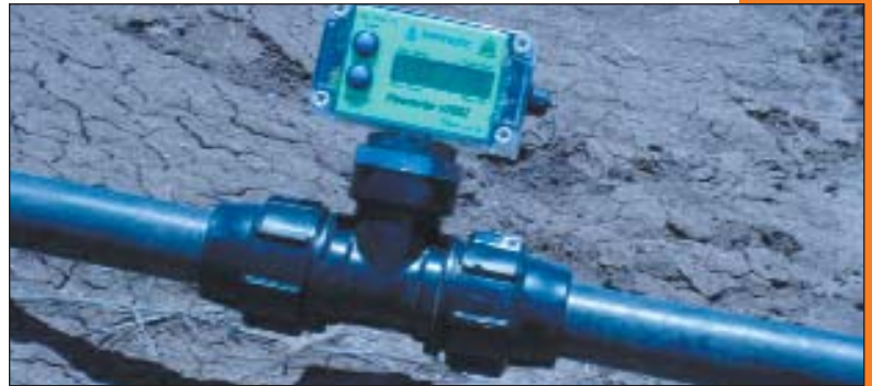
Flow meters in siphons provide vital information.
