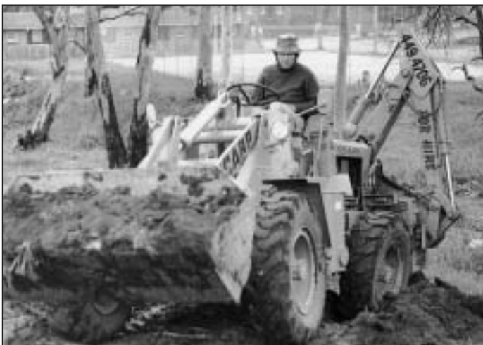
An FL 70 being put through its paces in outer Sydney by operator Chris Wight of Wycarp Pty. Ltd. A two wheel drive conventional rig could not have handled these steep wet conditions. (Photo I.M.J.)
