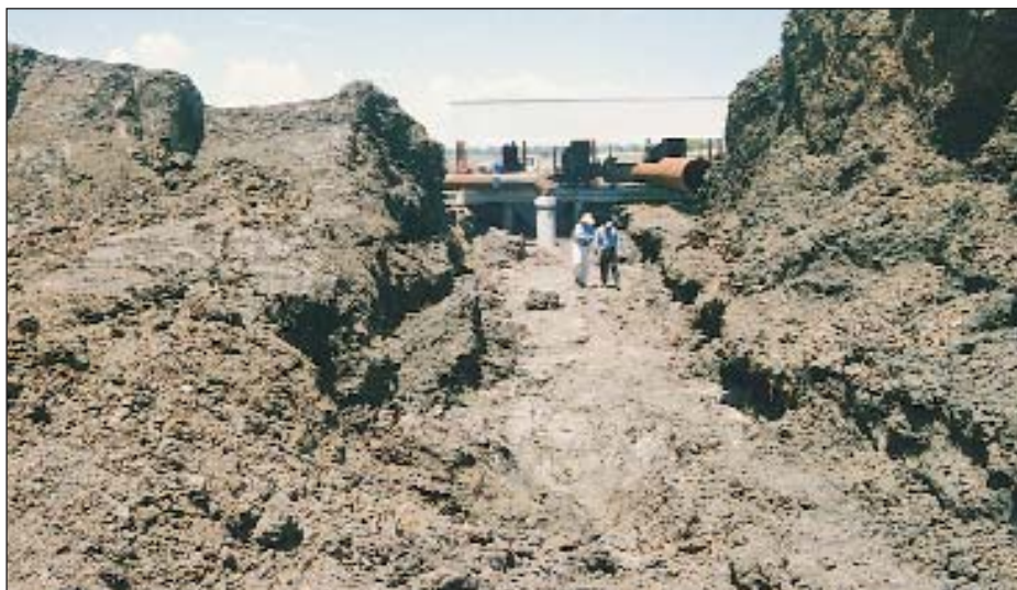
Bank failure along top of pipe through embankment to pumping station. Special care is needed when compacting around pipe. Cut-off collars, preferably flexible, should be installed around pipe
