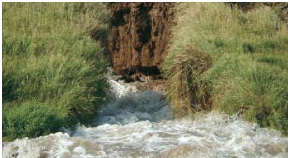
Vigorous grass over the whole embankment. Note cracked blocking structure in the embankment from grass roots.
