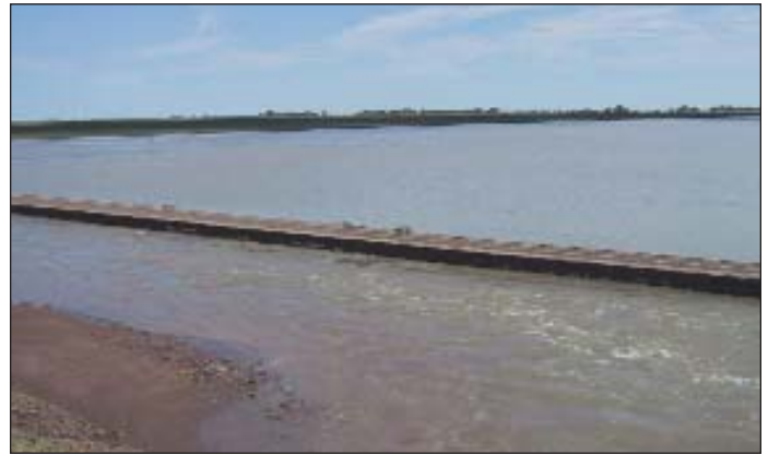
Physical damage outside the embankment is generally relatively small but crop damage from water can be a problem.
