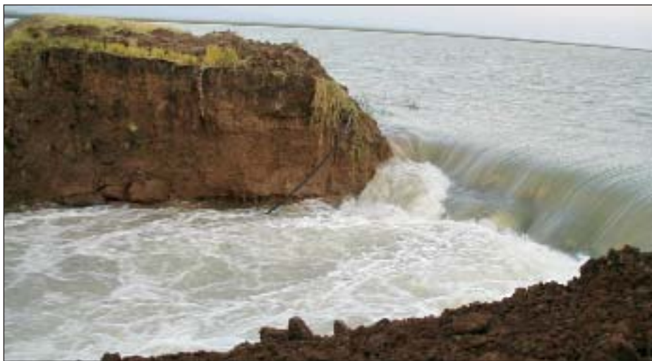
5.20pm: Once the water starts flowing through cracks, failure is quick and hard to stop.
