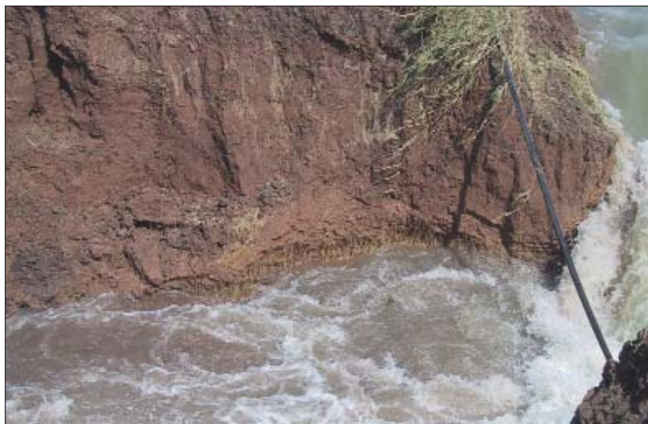
3.45pm: The early stages of a break in a storage wall — note the grass roots right through the embankment and the dripline for irrigating grass.
