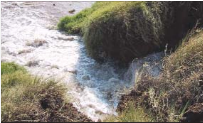
Grass on outside batter also growing into embankment with cracks coming from both sides.
