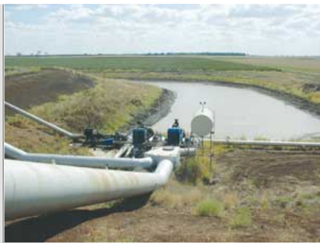
Recycled water could make a big contribution on the Downs.
