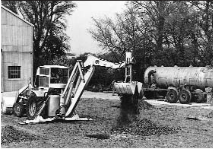
The Whitlock Dinkum 60 is shown with an optional clam shell attachment. In order to gain stability when using the clam shell or a large trenching bucket, the wide stabilisers were a necessity to prevent the tractor tipping when a full bucket was slewed to right angles in preparation for dumping. However the design of the stabilisers prevented the backhoe digging a parallel trench close to a wall or obstruction. Note the trapezium boom linkage. (I.M.J. archives).
