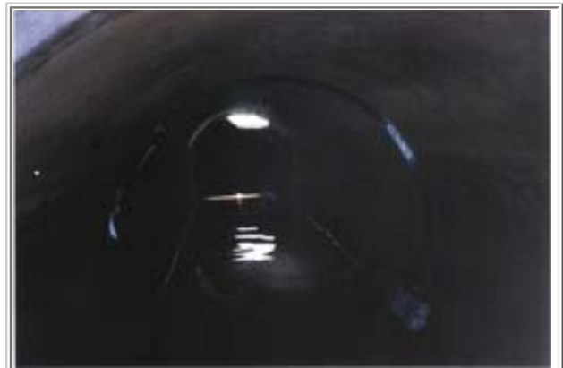
Starflow flow sensor in-situ in a concrete pipe
