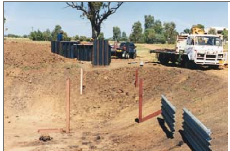
The earthworks for the new permanent irrigation display by BMC have created a lot of interest along the Newell Highway.
